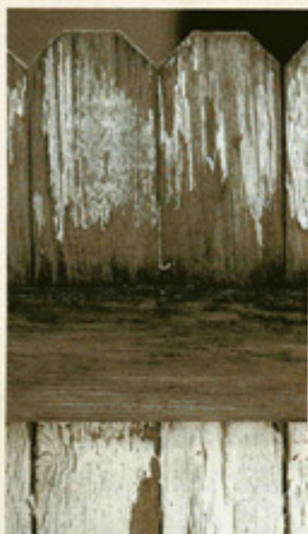
Wood rots and can require a great deal of maintenance.
